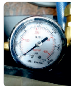
Pressure Gauge to monitor Water Output
